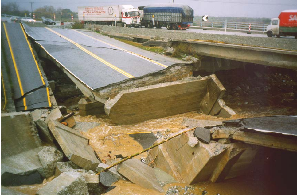
Figure 1. The Ziliana bridge afterwards the destruction. The circulation has been diverted on the new bridge of the right lane of the motorway Athens–Thessaloniki.
