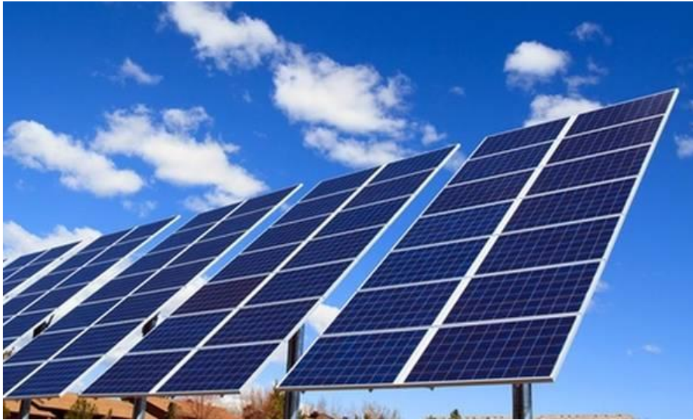
Figure (I.3) : panneaux photovoltaïques. [24]
