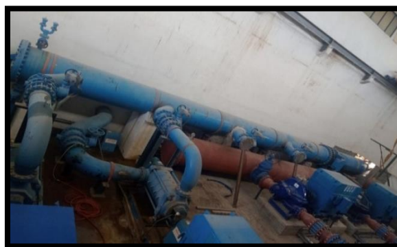
Figure III. 4: Station de pompage SP1
