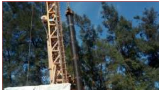
Figure 25: Mât de forage
