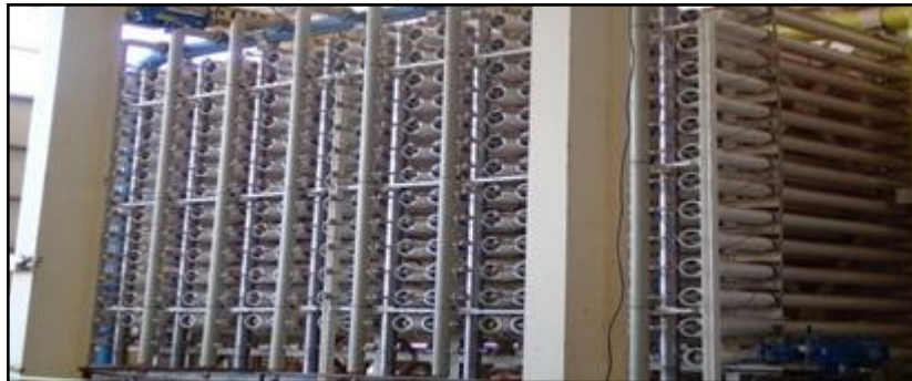
Figure III. 7: Rack d'osmose inverse
