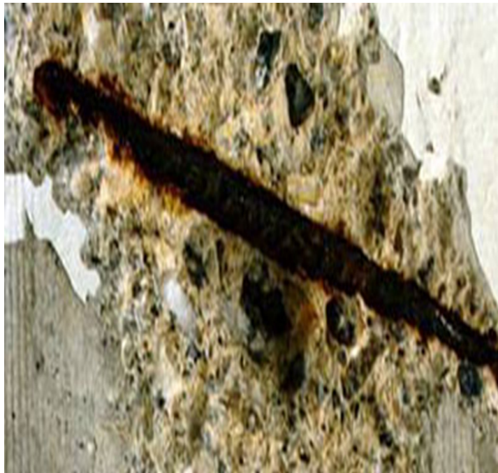
Figure [2.5] - corrosion des armatures
