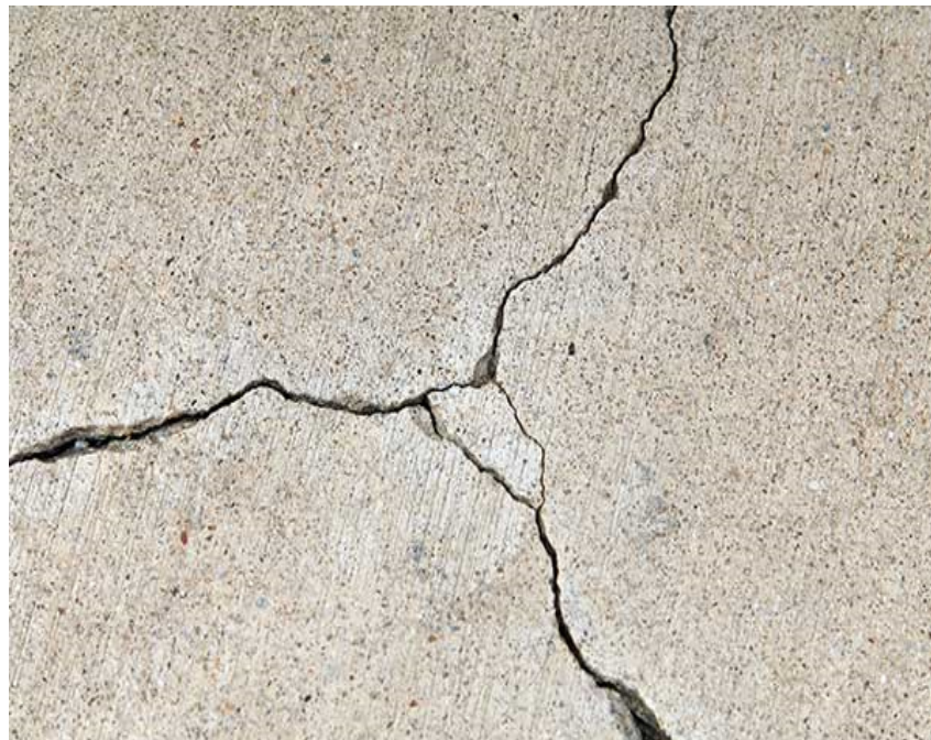
Figure [2.1] - fissuration du béton
