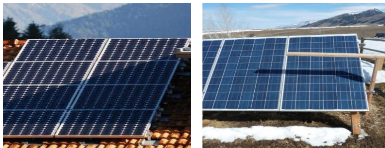
FIGURE 2.10 – Modules photovoltaïques ombragés
