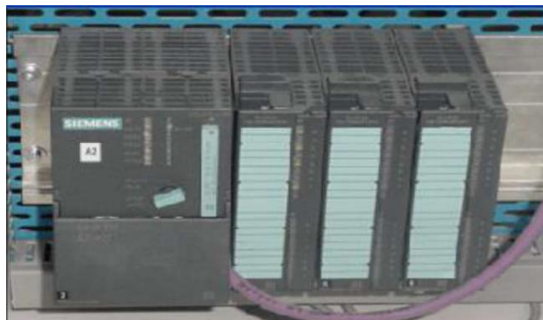
Figure I.12 – Automate programmable industriel. [8]
