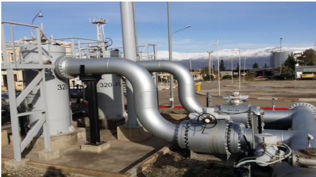
Figure 1.4: Les Filtres de la station SBM.
