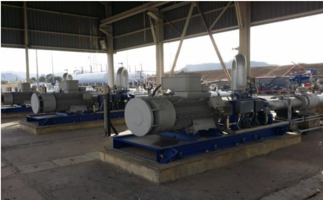
Figure 1.6: Les pomperies boosting.
