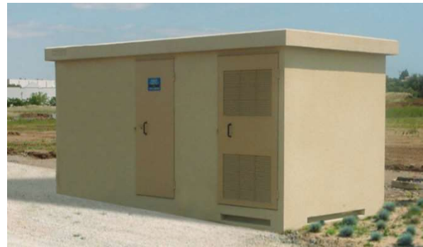
Figure I.6 : poste de transformation [11]
