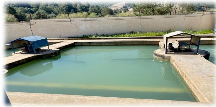
Figure II. 6: Bassin de floculation
