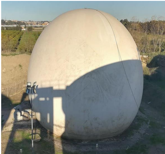
Figure II.9: le stockage du biogaz
