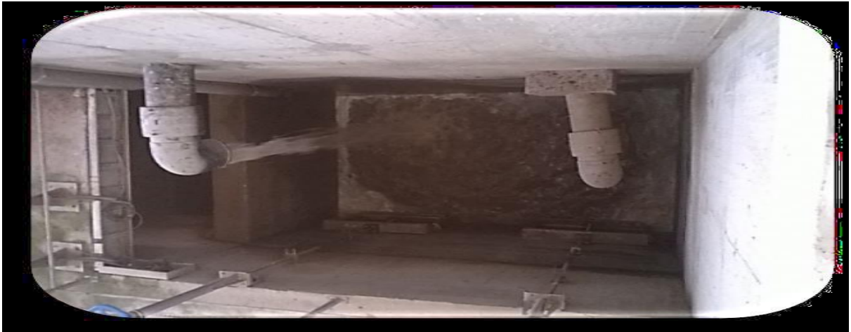
Figure 7: La tête de la station
