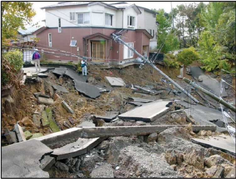
Figure I.3. Earthquake-induced landslide damage to a house built on artificial fill, after the 2004 Niigata Prefecture earthquake in Japan. [1]
