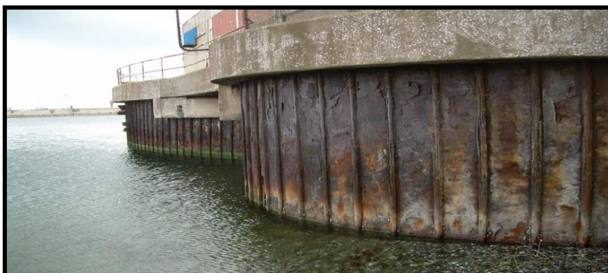
Figure I. 36: Corrosion de palplanche.
