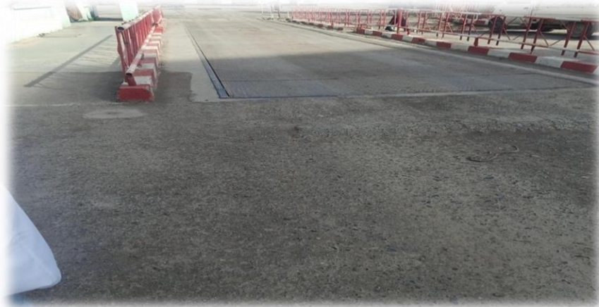
Figure 4 : Pont-bascule apparent (photo original)
