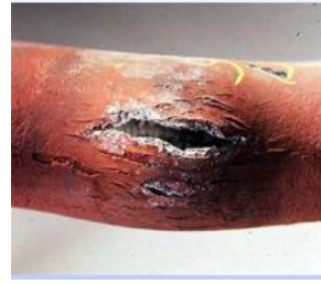
Figure I-19 : rupture de tuyau
