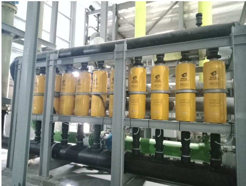
Figure III.13: Installation of pressure exchanger
