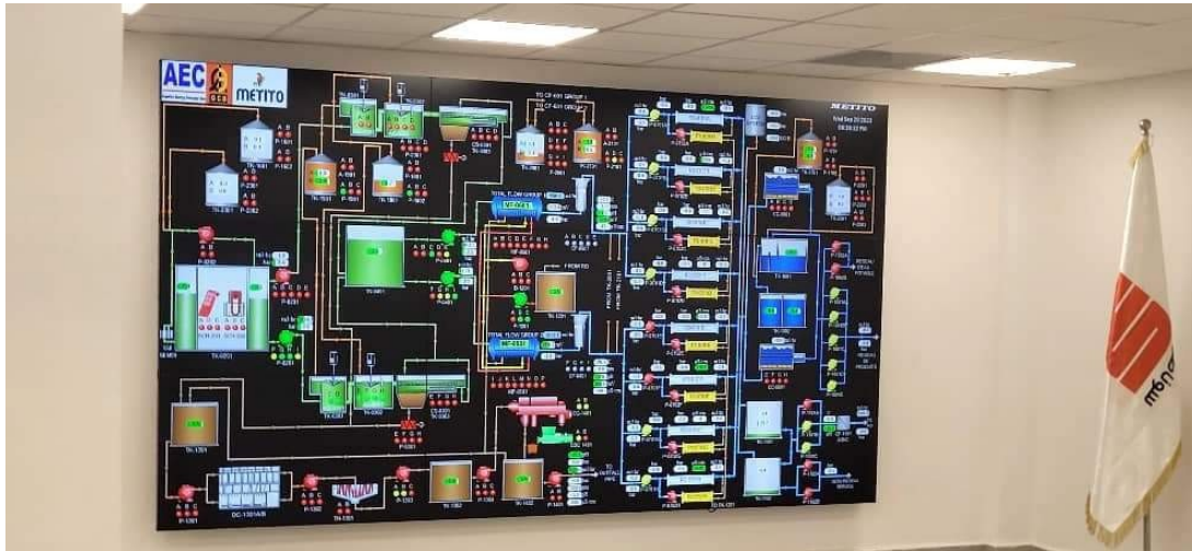
Figure III.15: The control room
