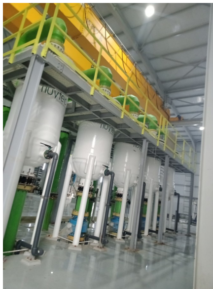
Figure III.10: Installation of cartridge filters
