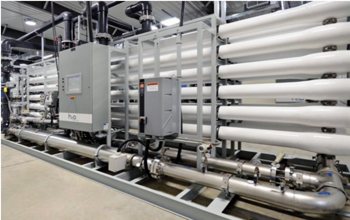
Figure III.12: Reverse osmosis units
