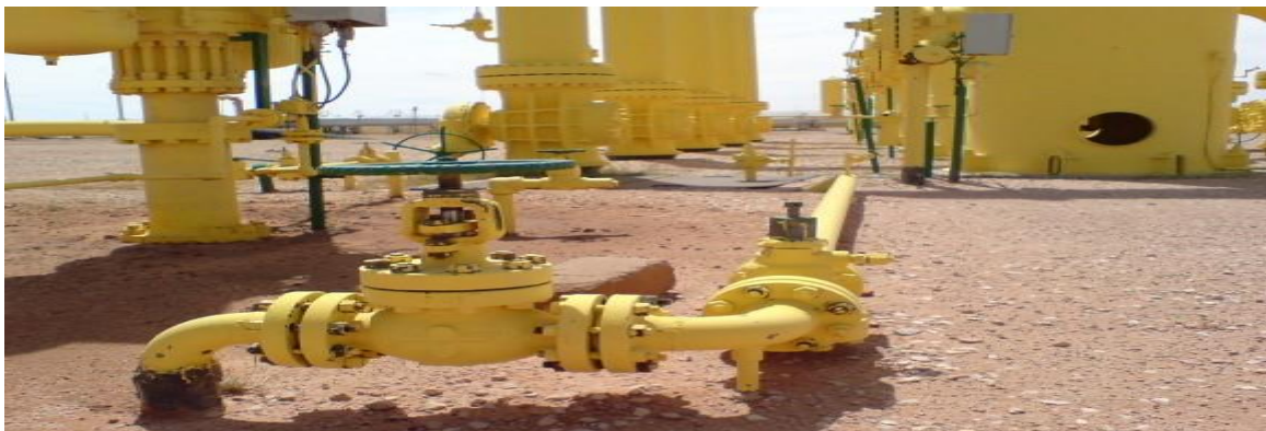
Figure III- 3 : Vanne Entrée Station GOV 2045
