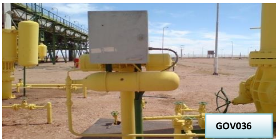
Figure III-1: Vanne Alimentation Skid Gaz
