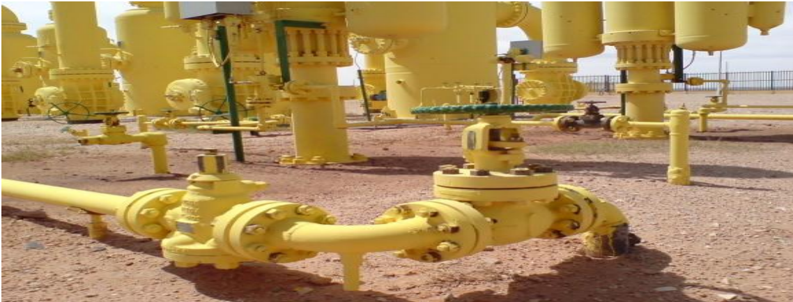
Figure III- 4 : Vanne Sortie Station GOV 2046
