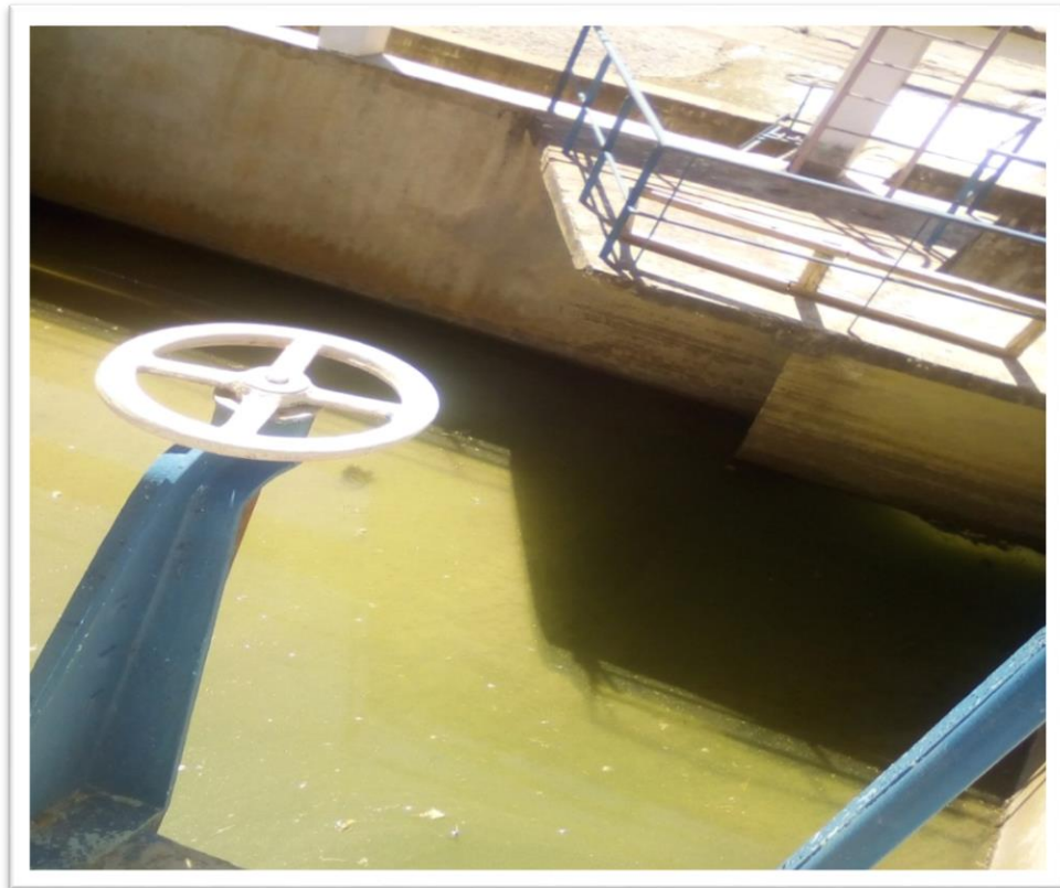
Figure 07: Chambre de relevage
