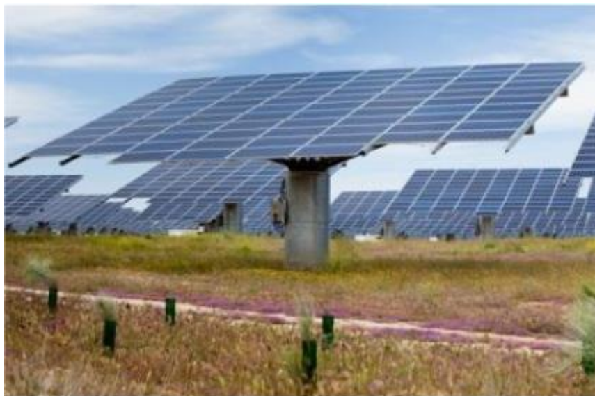
Figure (I.1): Panneaux solaire photovoltaïque
