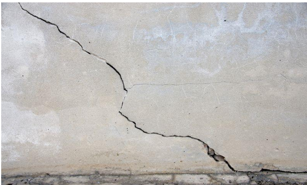
Figure .I. 1 : Fissuration
