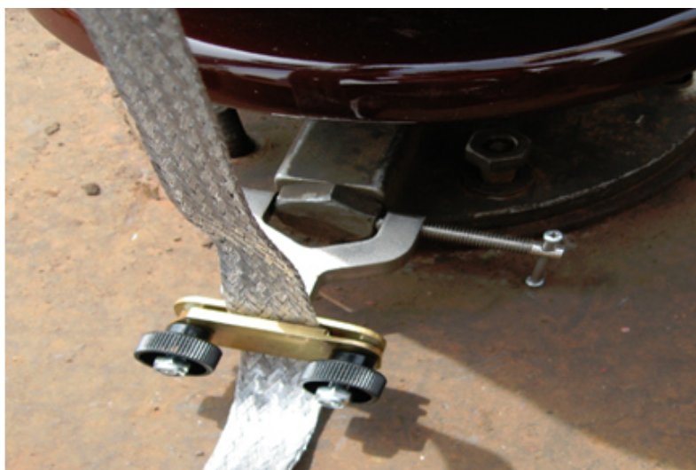
Figure III.8: Raccordement de la terre au FRAnalyzer.
