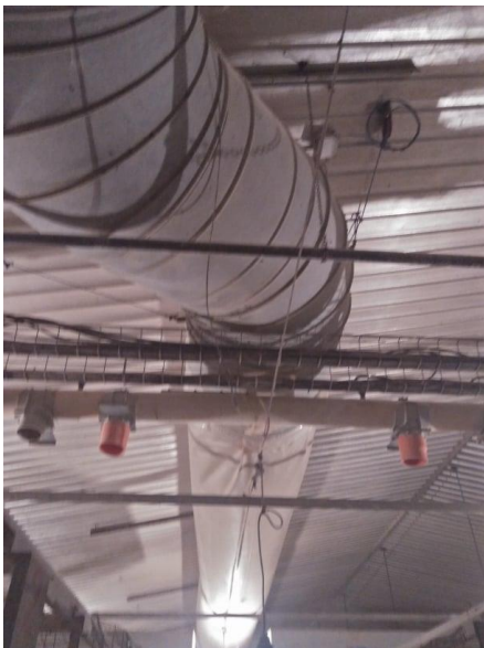
Figure 20: Chauffage a air pulsé (Photo personnelle, 2020).
